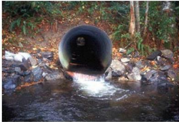
Figure 21. Round, corrugated metal culvert retrofitted with corner baffles to improve fish passage
