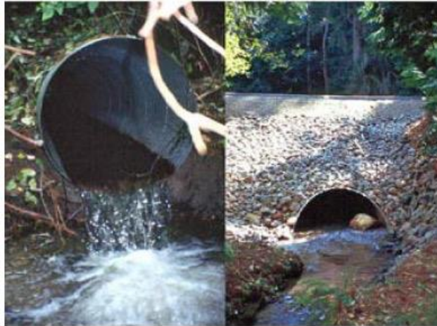
Figure 24. Undersized perched culvert (left) replaced with larger pipe designed using stream simulation option
