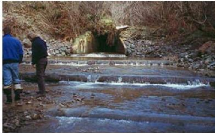
Figure 19. Series of channel spanning weirs used to step up water surface and raise outlet pool to culvert lip
