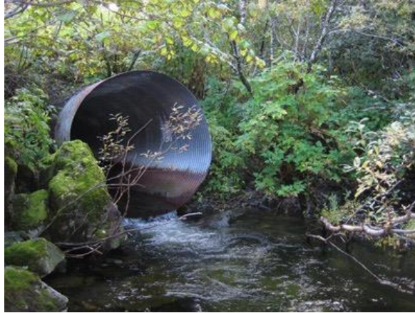
Figure 18. A significantly perched culvert
